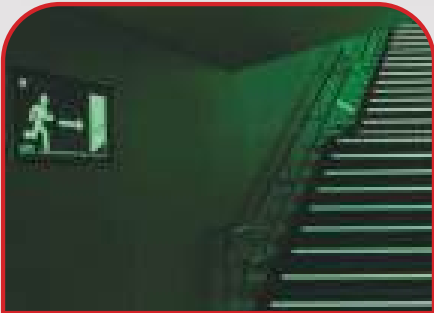
Low Location Lighting
