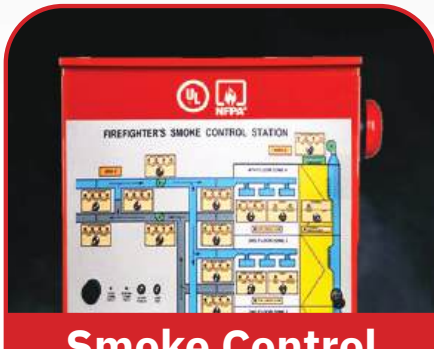
Smoke Control Stations
